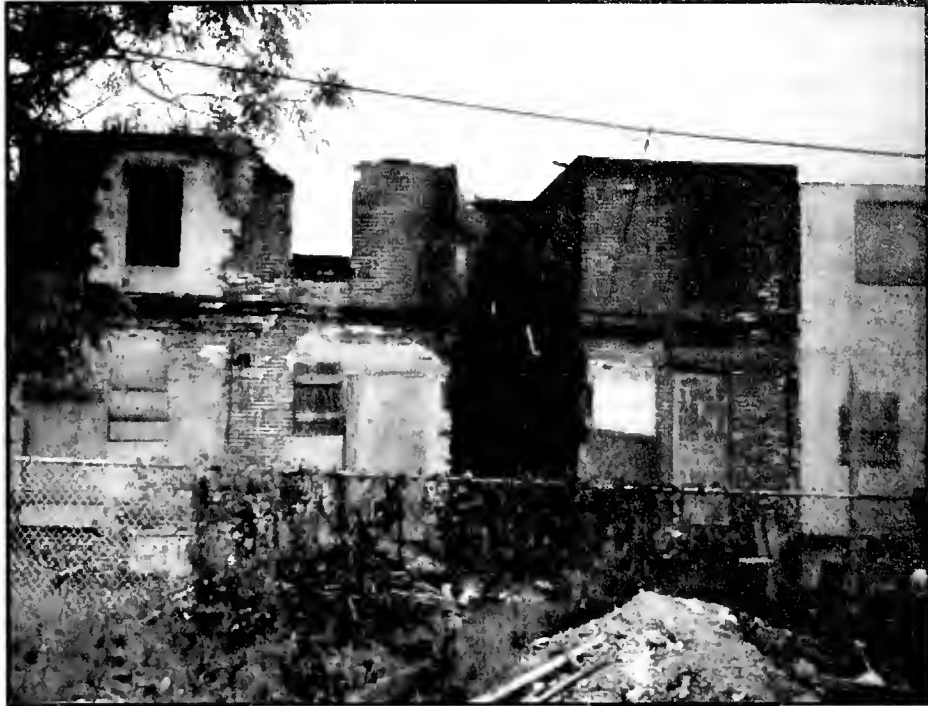
Figure 8: Rear view of south side of Clinton Street before rehabilitation. Photo courtesy of Metro Camden Habitat for Humanity.
